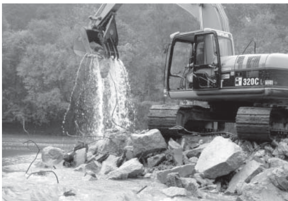
A bulldozer clears rubble during the removal of Marvel Slab on the Cahaba River. Photo by Paul Freeman.
